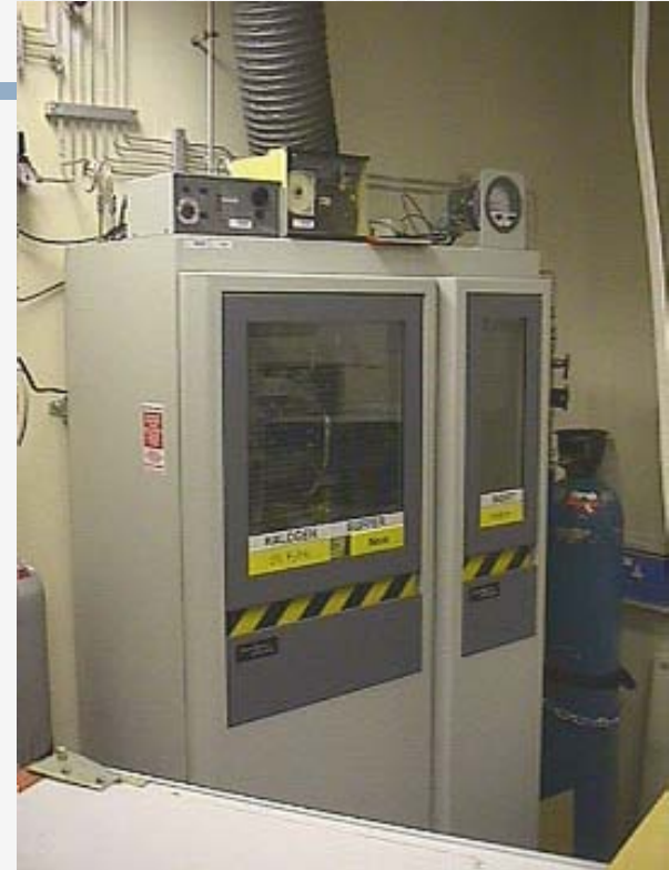
Total Enclosure – Ventilated Cabinet for a fluorine gas cylinder
